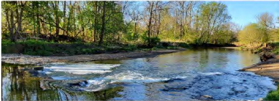
FIGURE 9: J-hook og vane designed and installed (May 1, 2019) on Eagle Creek by FLR & ESE
