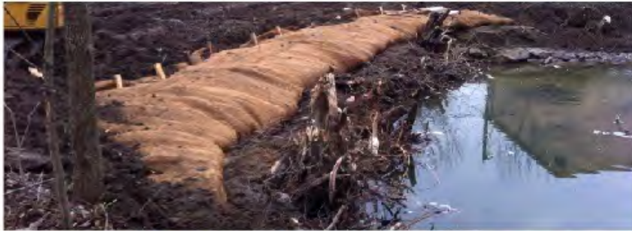
FIGURE 8: Root wads designed and installed (Dec 2, 2011) on Payne Branch of Crooked Creek by FLR
