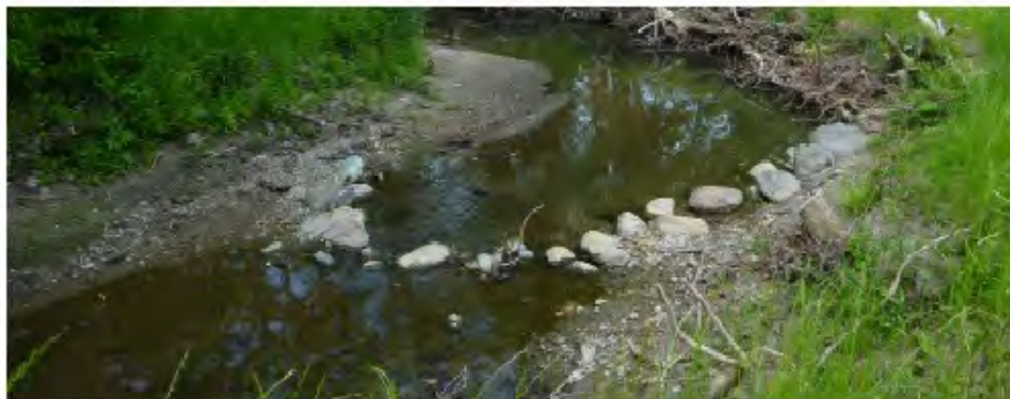
FIGURE 10: Cross vane designed and installed (Nov 23, 2011) on Payne Branch of Crooked Creek by FLR
